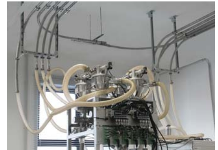
Overhead photo of OCS pellet transport system
